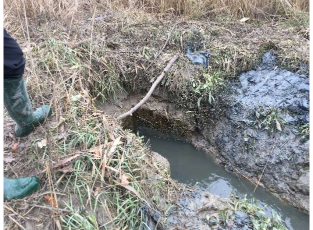
The culvert running through the sea wall, draining into the tidal river.
